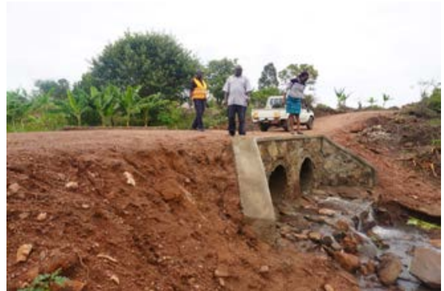
Works Committee Chairperson Hon. Leku Gloria, the Secretary of Social Services, and Engineer Afimani Simon inspect the newly built culvert on the Anguru-Ejupala road, a key component of ongoing efforts to improve connectivity in West Nile.
